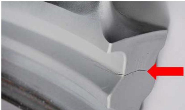
Incipient crack in an LP end blade after a very short operating period due to excitations from an unfavourable steam current
